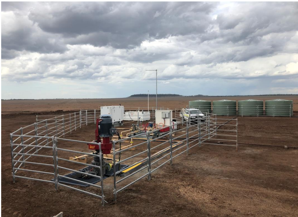
Figure 1 – Production testing equipment at the Memooloo 2 vertical well.
