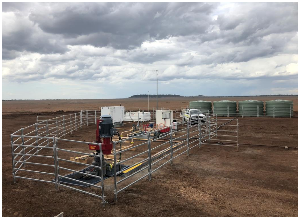
Figure 2 – Production testing at the Memooloo 2 vertical well with water storage tanks in the background
