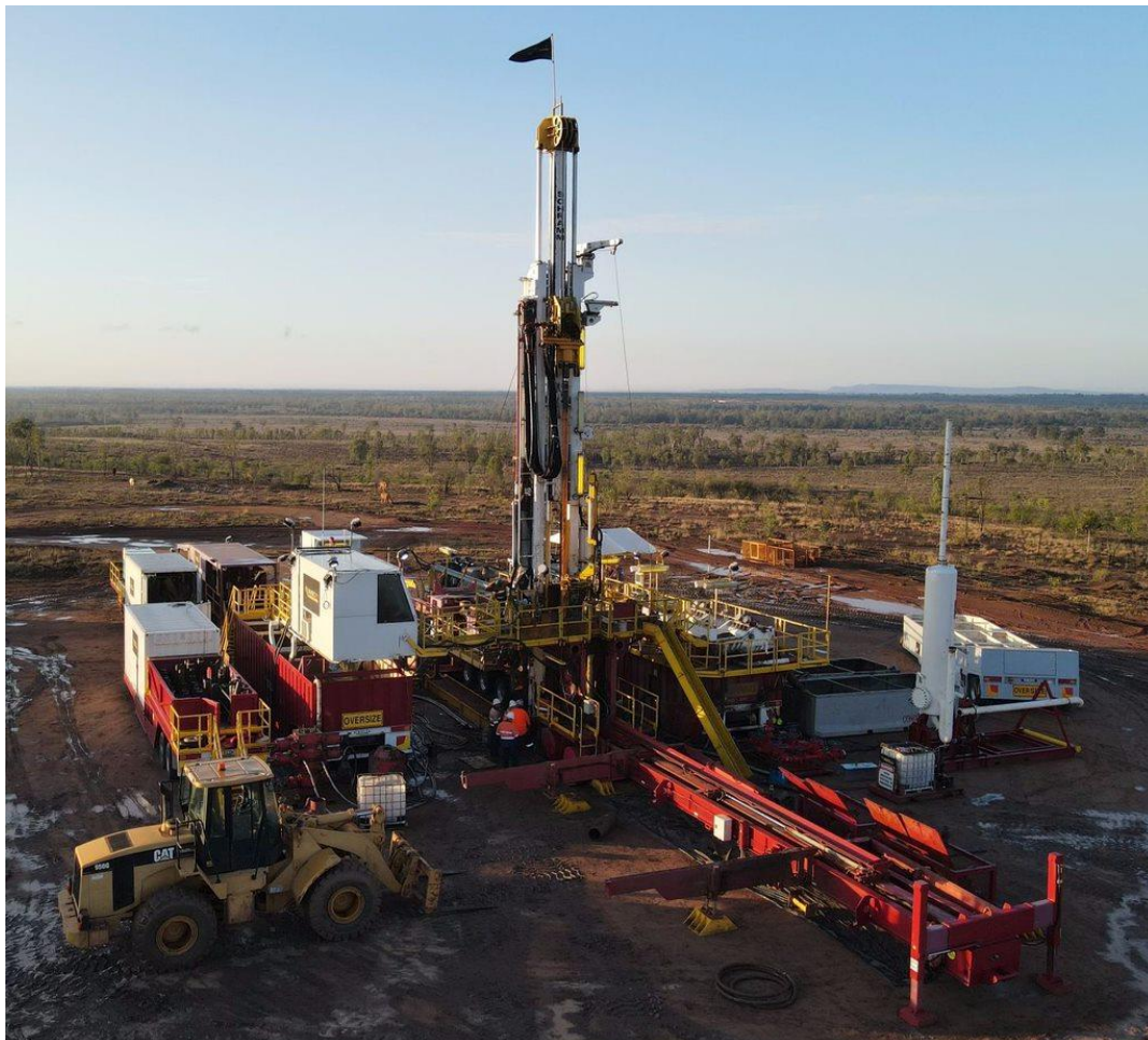
Figure 4 - Silver City Rig 23 in the process of rigging up on the Mahalo North 2 location in ATP 2048
